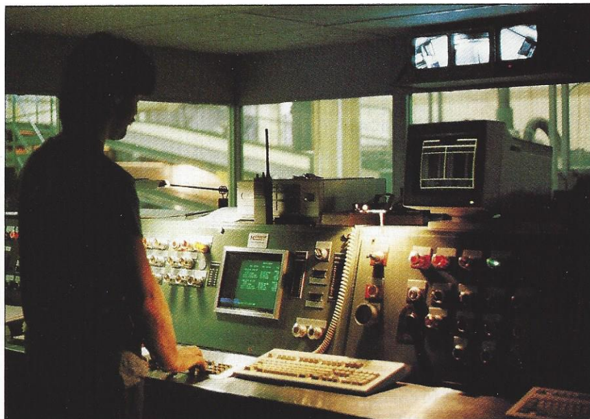
The Marquip Data Master 3 is located in the corrugator control room at Great Northern. Information from the Corr-Trim scheduling system is downloaded to the Data Master and, through that, into the Marquip equipment, the Copar wet-end computers and the Pentek conveyor computers.
