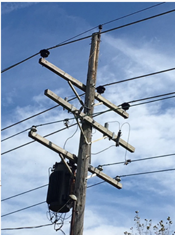
A lightning strike on this pole momentarily interrupted power to part of the Argonne site. Near the top of the pole, the lighter, unweathered wood was exposed where the lightning hit.
